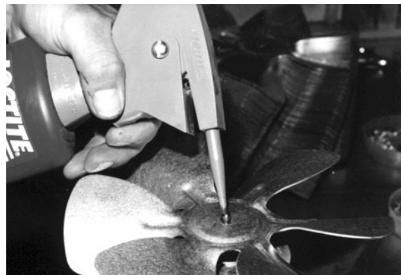
Loctite® 271™ Threadlocker is used to fasten down the cooling fan blade retaining nut.
